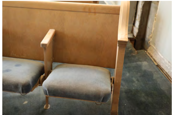
Figure 41: Accumulation of dust and dirt on theater seating upholstery in the Auditorium (Room 107)
