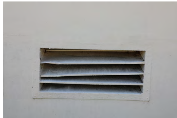
Figure 11: Damaged fins of the louver at the north elevation
