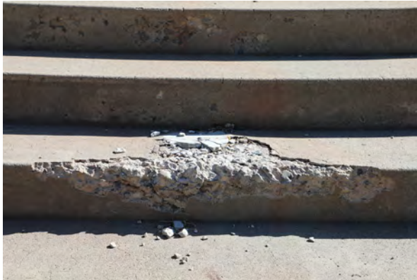
Figure 03: Significant deterioration of the concrete steps at the southwest stair
