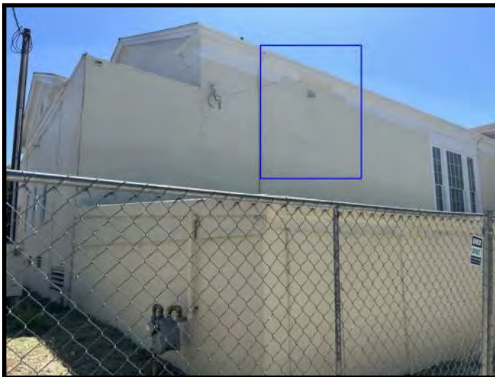
Figure 30 View of bubbling plastic membrane at the west exterior wall.
