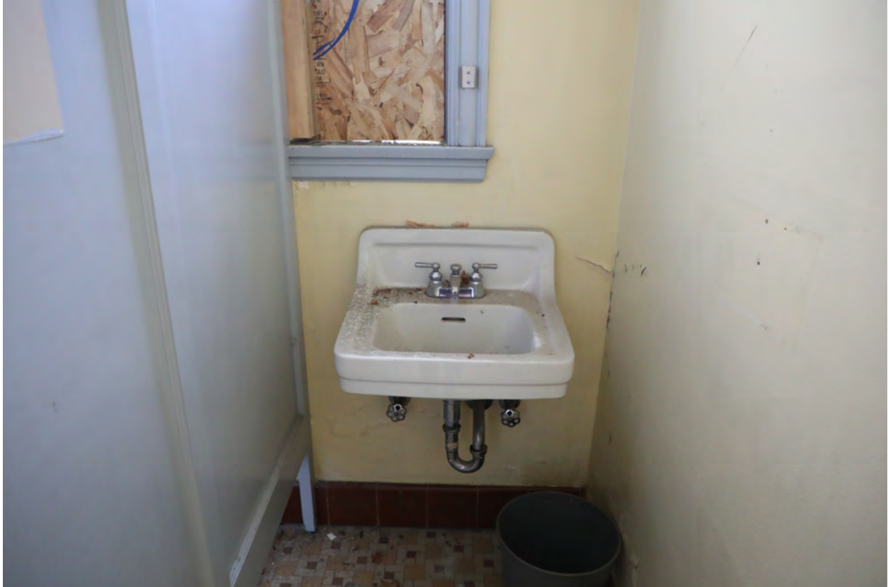
Figure 21 - 1st floor mens restroom, looking at window and sink, view north (ARG, 2024)
