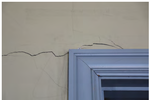
Figure 36: Significant cracking of plaster at cased opening on the north wall of west Lobby (Room 115)
