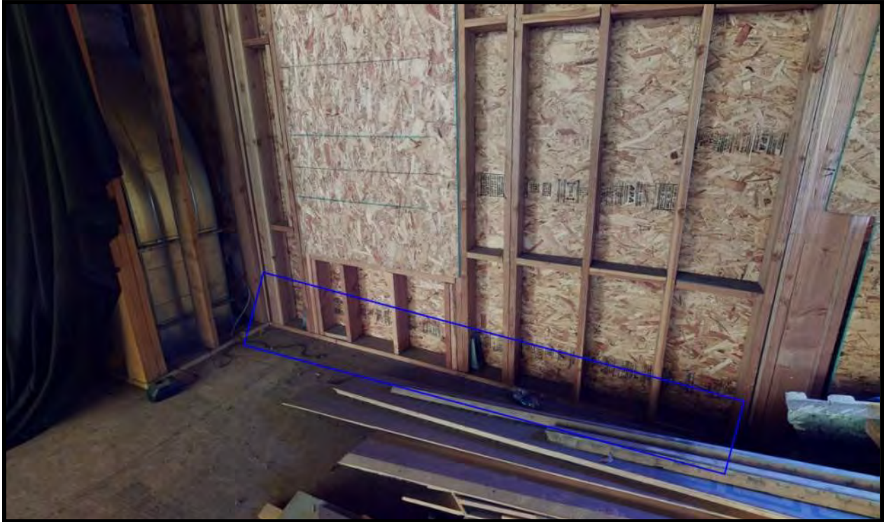
Figure 28 View of missing sill bolts at the north wall of the stage.
