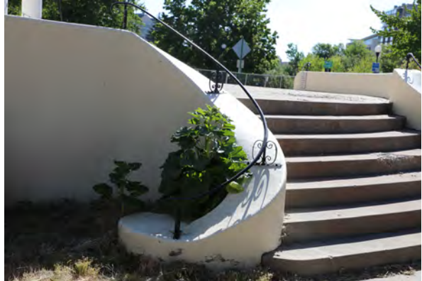
Figure 02: Non-compliant handrails at the southwest stair
