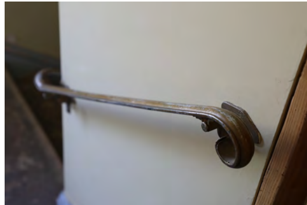
Figure 40: Stair handrails lack ADA compliant extensions, and are not at the proper height
