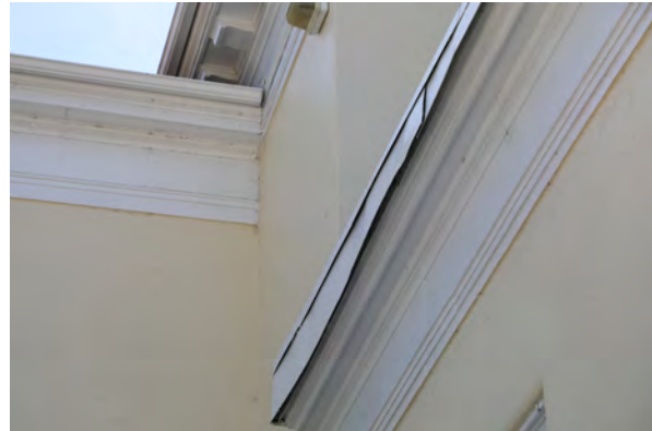
Figure 07: Unsecured sheet metal flashing at north wall of the west wing
