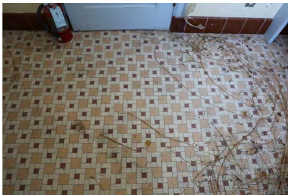
Figure 33: Dirt accumulation at original tile in Women's Restroom (Room 112)
