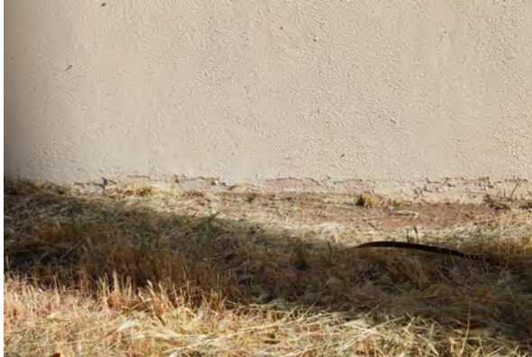
Figure 01: Deteriorated paint at the base of the exterior stucco walls along the south elevation
