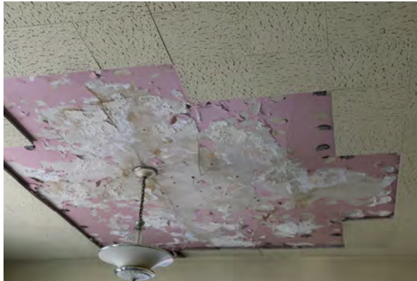
Figure 37: Missing acoustic tile and damaged historic finish at ceiling of the Literature Room (Room 114)
