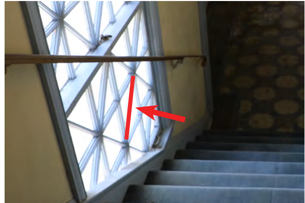
Figure 16: Missing interior muntin at Window 1-12
