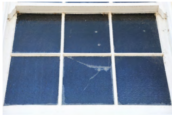
Figure 18: Damaged glazing at Window 1-01 on the north wall
