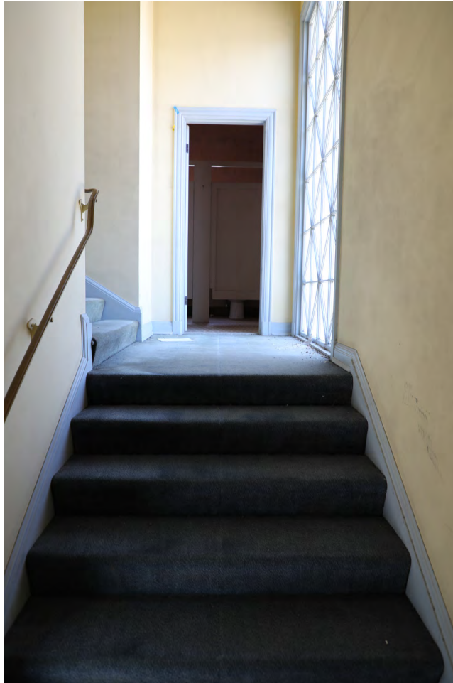
Figure 34 - Stairs to balcony looking from first landing, toward women's restroom, view north (ARG, 2024)
