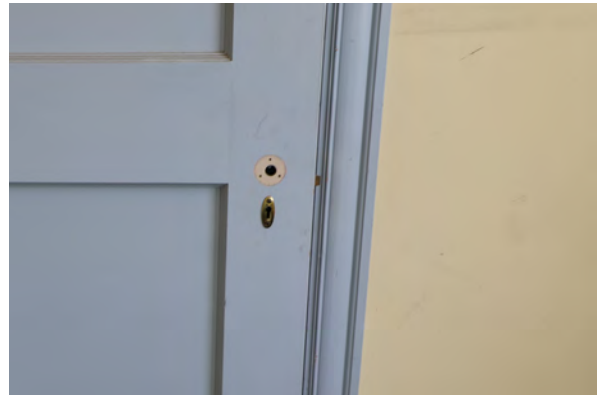
Figure 28: Missing hardware at Door 1-05
