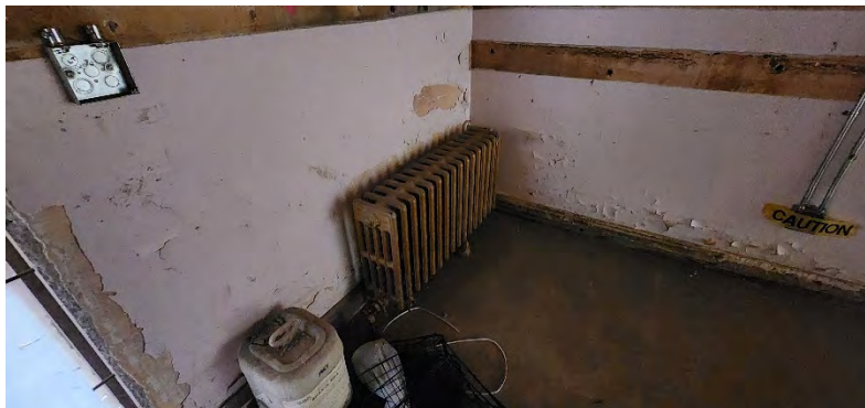
Old steam radiator:
