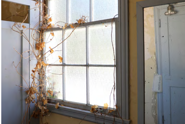
Figure 19: Ivy growth at window 1-20 in the Women's Restroom (Room 112)
