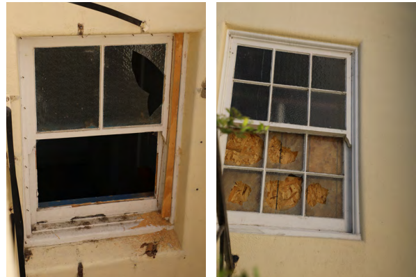
Figure 17: Damaged sash and broken or missing glazing at Windows 0-10 (left) and 1-10 (right)
