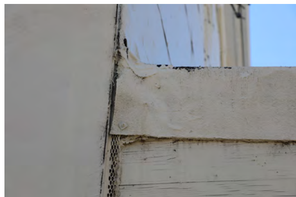
Figure 12: Exposed stucco lath between northwest addition and the temporary wall and roof of the unfinished west addition
