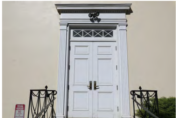
Figure 23: Exterior flood light at the East Entry
