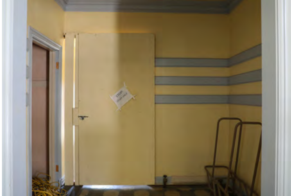
Figure 25: Makeshift plywood door in Lobby (Room 103) and missing door to Closet at the left
