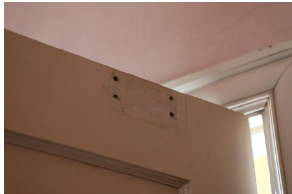
Figure 29: Missing door closer at Women's Restroom, Door 2-01
