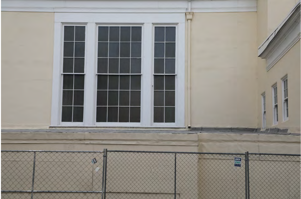
Figure 14 - West facade, looking at large window above temporary structure enclosing incomplete 2002 addition (ARG, 2024)
