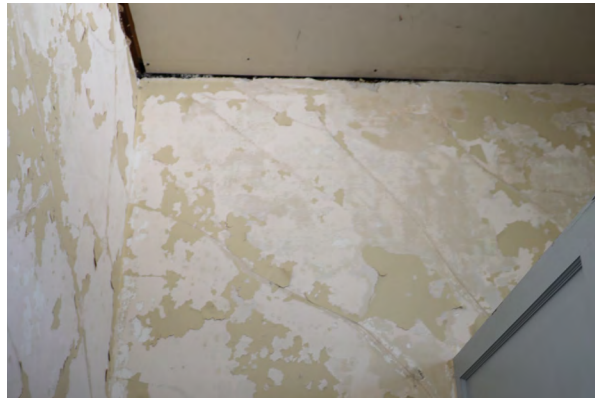
Figure 35: Severely damaged paint finish and plaster, possibly caused by ivy removal in the west Women's Restroom (Room 112)
