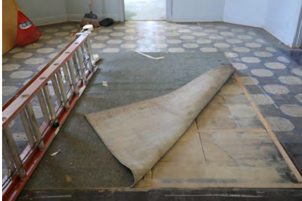
Figure 31: Fire damaged and missing vinyl tile under a temporary carpet section in the west Lobby (Room 115)
