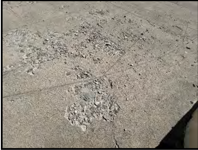
Figure 24 View of spalling slab-on-grade at the south entrance to the theater.
