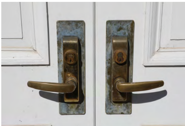
Figure 15: Tarnished hardware at east entry (Door 1-04)
