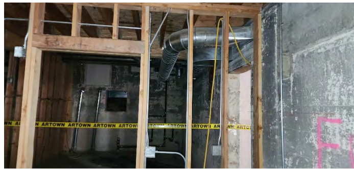
Existing ductwork in basement:
