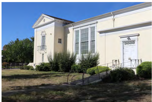
Figure 06: Non-compliant ramp and sidewalk overgrown with vegetation at the east entry
