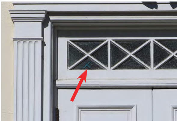
Figure 14: Cracked glazing at east entry transom
