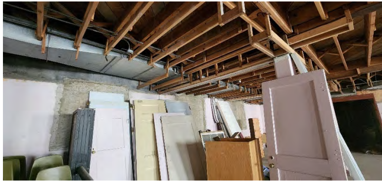
Circa 1934 existing ductwork:
