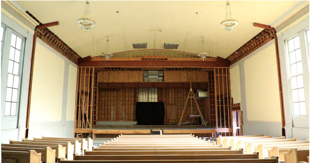
Lear Theater auditorium showing new stage and steel framing, view north (ARG 2024)
